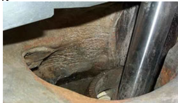
Rust hole found in the reactor's carbon steel lid in March, 2002.
