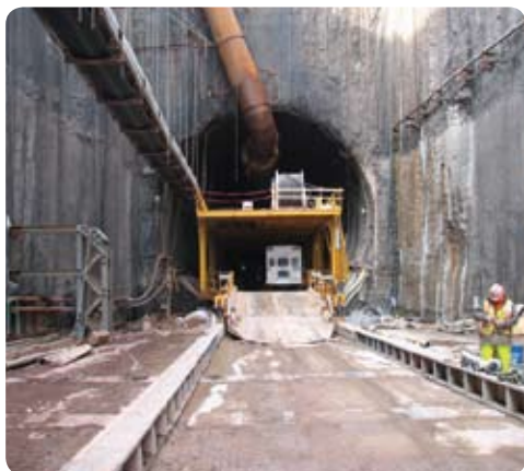
The entrance to the Niagara Tunnel, going under the city of Niagara Falls. The Tunnel’s distance has been reduced by about 200 metres due to an alignment revision – shortening its length from 10.4 kilometres to 10.2 kilometres.
